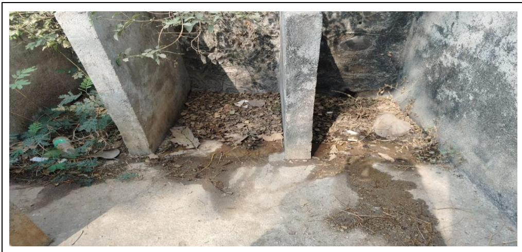
Figure 2 : Unclean and open bathroom at Dnyandeep Boys Hostel, Belora, Mantha, District-Jalna
