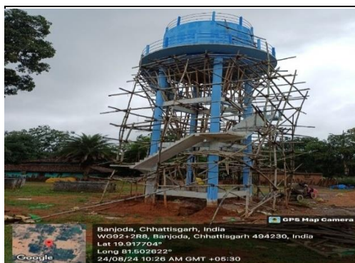
Photo 4.6: Incomplete OHT at village Banjoda, District: Kondagaon
