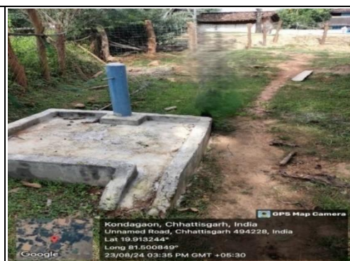
Photo 4.7: Non-functional household tap connection at village Banjoda, District: Kondagaon
