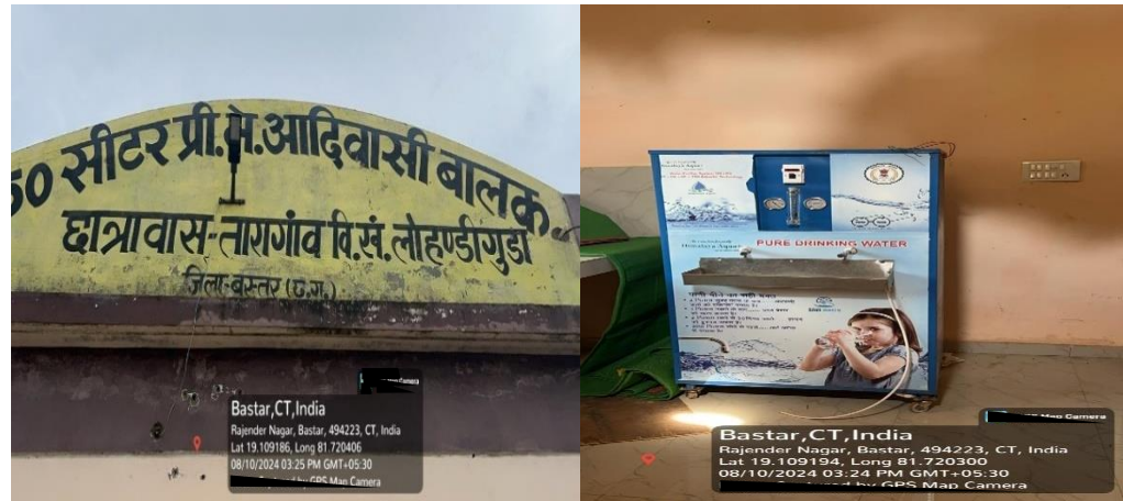
Picture 3.11: RO systems supplied in tribal hostels of Bastar district, was not in working condition and the Hostel Superintendent reported that the candles of the RO purification systems had not been cleaned or serviced since their installation.
