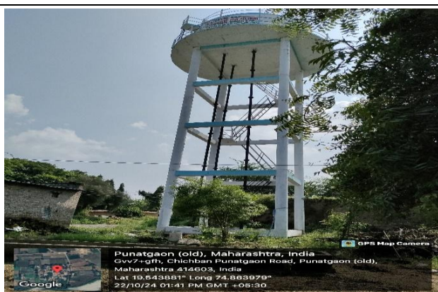
Photograph 7: ESR without fencing at Village Punatgaon Block: Nevasa
