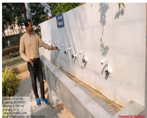
Photograph 17: Chamakhandi HS: No water supply at MTMC
