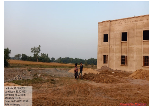
Photo No. 8: Construction of 180 capacity male ward of Bhadrak jail without outer jail wall
