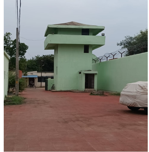
Photo No. 11: Watch tower without any personnel or security equipment, Special Jail, Bhubaneswar
