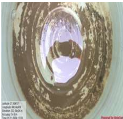
Photo 5: Polluted water in overhead tank used in Barmal AWC for drinking and cooking
