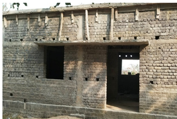
Photo 6: Non-completion of AWC building under MGNREGS in Phalsadhipa
