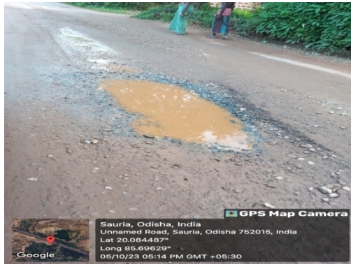
Photo No-6: Non-executed portion of Pattanaikia-Delang-Khordha road with big potholes (Khordha R&B)
