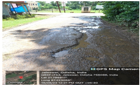
Photo No-5: Existence of SL road in the entry point of Jaleswar to Paschimabad from 0/000 to 1/900 km due to non-improvement /widening of road (Balasore R&B-II)
