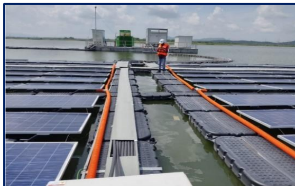
Figure 4.3 - NTPC Ramagundam Floating Solar Plant
