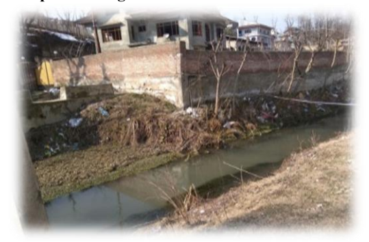
Earth filling in Bata Khul and waste material dumped on fringe of nallah
