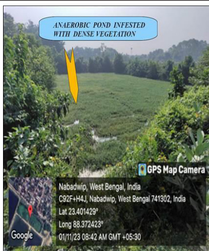
Figure 4.7: Anaerobic Pond infested with dense vegetation
