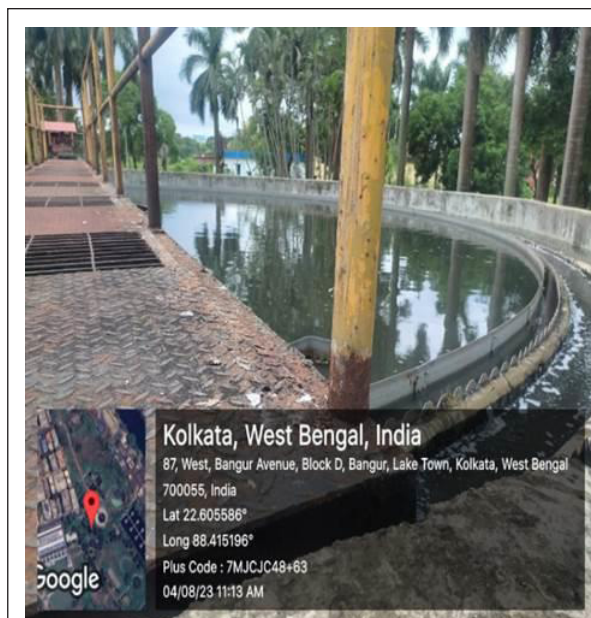
Figure 4.16: Primary Clarifier at the STP
