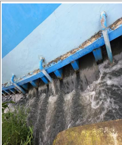
Figure 4.17: Treated water discharging into outlet drain
