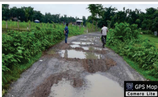
Fig. 4.15: Big size potholes filled with rainwater
