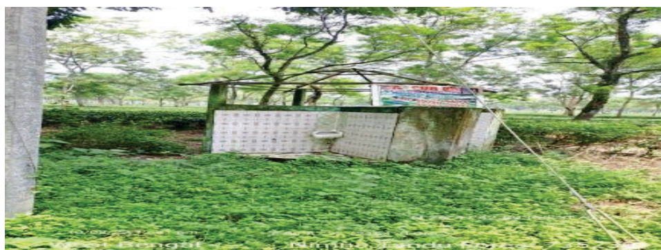
Fig. 3.29: Dilapidated condition of Toilet at Gorumara Forest, Jalpaiguri
