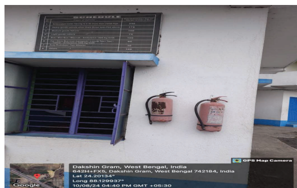
Figure 2.10: Picture showing rusted and expired fire-fighting devices
