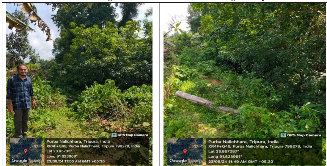
Photograph 2.2.17 and 2.2.18: Status of Village link road for Community from Old Bhudda Mandhir to Kachimchara road under Basudeb Para GP
