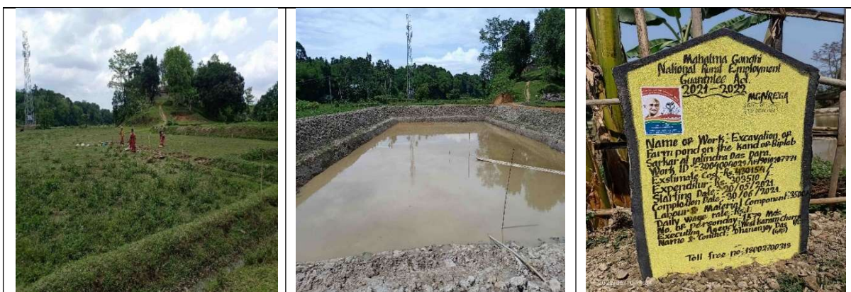
Photographs 2.2.24, 2.2.25 and 2.2.26: First stage, second stage and third stage for excavation of farm pond on the land of Biplab Sarkar at Jatindra Das Para under West Karamcheera VC during 2021-22, expenditure: ₹ 3.04 lakh
