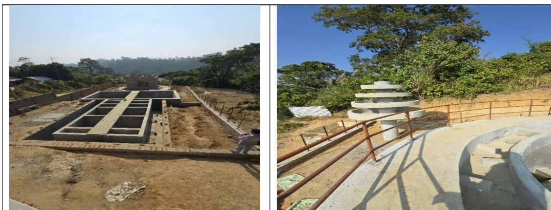
Photographs 2.3.9 and 2.3.10: Incomplete Innovative scheme at Manoranjan Para, Magroom VC under Rupaichari Block of South Tripura District
