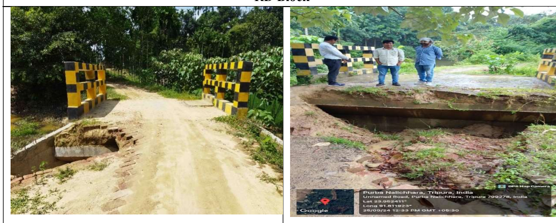
Photographs 2.2.3 and 2.2.4: Washed away part of the brick soling road, first photo during construction of the box culvert obtained from Bhuvan App and second photo as noticed in the JPV
