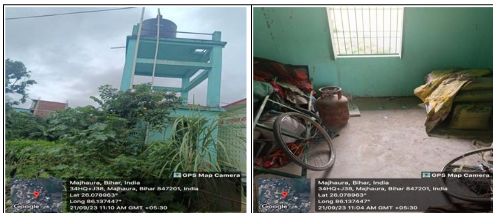
Water supply scheme (left side) and non-installation of IRP in pump house of water supply scheme (right side) in ward no. 17 of Benipur NP, Darbhanga
