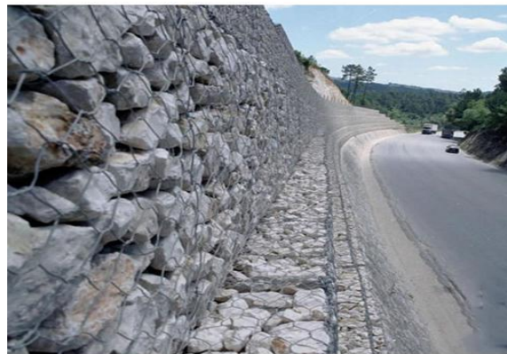
Photo No.29 - Use of Gabion Boxes as retaining wall in road works
