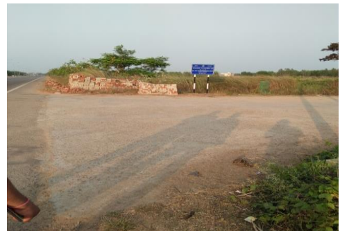
Photo No.32: Completed portion of road - Khandia Bandha to NH by-pass (NH-316)
