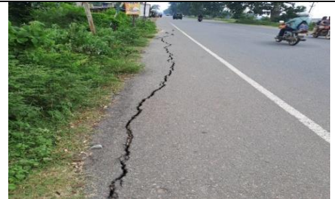
Photo No. 20: Liner and crocodile crack from Km 30/000 to Km 35/000
