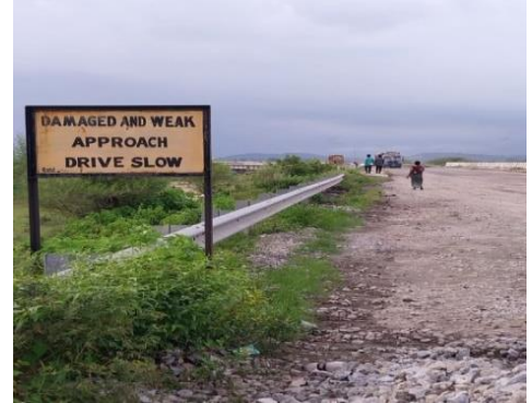
Photo No. 19: Damaged and weak approaches of 4 bridges
