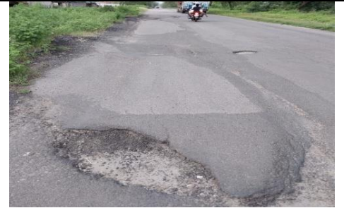
Photo No. 18: Depression at Km 26/125
