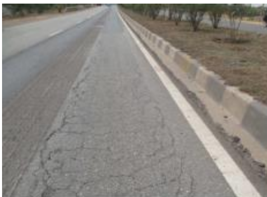
Photo No.14: Crack in BC at RD 73.300
