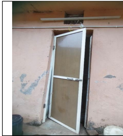
Photograph 3.1.6: Broken door of toilet of the STGH at Dogharia, Nuagada Block, Gajapati District
