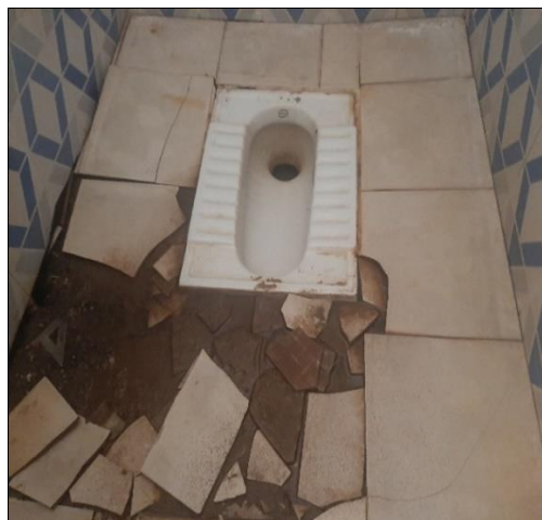
Photograph 3.1.18: Latrine flooring, requiring repair, at STGH, Baidpur High School, Badasahi Block, Mayurbhanj District
