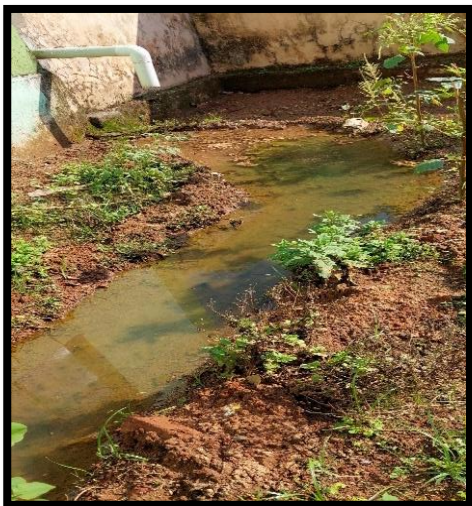
Photograph 3.1.10: Accumulation of waste water, due to lack of any drainage system, at the STGH, KC Pur, Guma Block, Gajapati District
