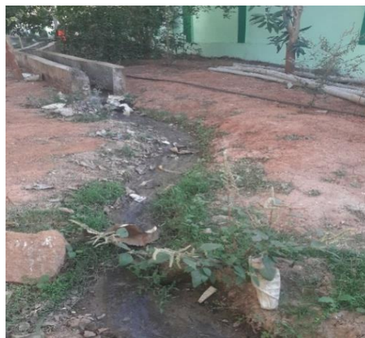
Photograph 3.1.11: Accumulation of waste water, due to partly constructed drainage system at the STGH, Tikabali HS, Tikabali Block, Kandhamal District
