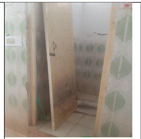
Photograph 3.1.19: Latrine door broken at STGH, Singarpur, Jashipur Block, Mayurbhanj District
