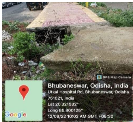
Photograph 8: Drain near Utkal Hospital, Bhubaneswar, showing no inlet and outlet provisions
