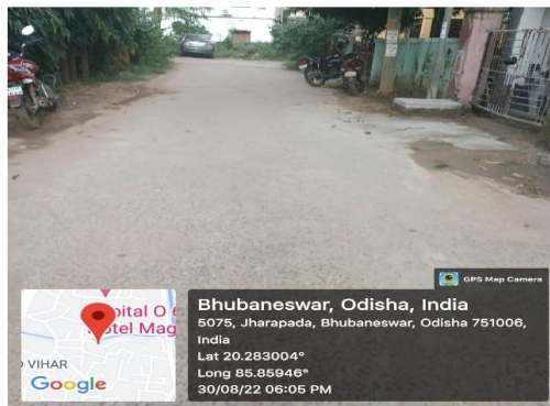
Photograph 13: Jharpada road near Drain No.7 having no drain facilities
