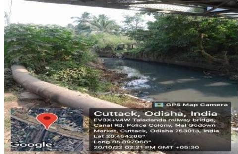
Photograph 19: Non-maintenance of Drain at Matrubhawan, Cuttack
