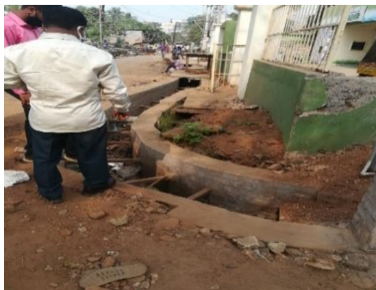
Photograph 7: Drain near Ashra, at Unit-III, Bhubaneswar, showing no inlet and outlet provisions
