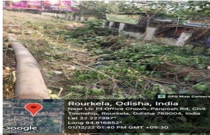
Photograph 20 : Non-maintenance of Drain at Raghunath Palli, Rourkela
