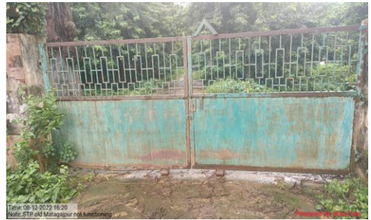
Photograph 48: Idle STP of 33 MLD capacity, at Matagajpur, Cuttack
