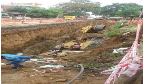
Photograph 26: Haphazard work at the Sambalpur sewerage project
