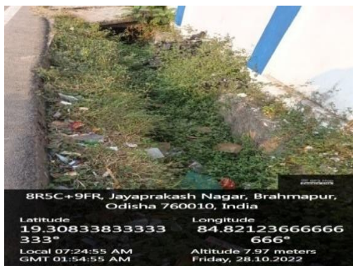
Photograph 16: Blockage of Drain at Jayprakash Nagar, Berhampur, due to unwanted vegetation and plastic waste
