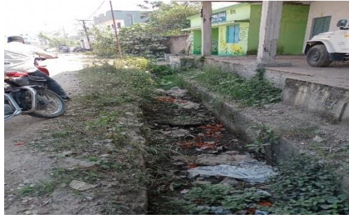
Photograph 18: Non-maintenance of Drain at Khetrajpur, Sambalpur
