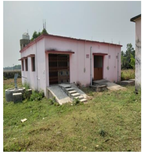
Labour room and Ward constructed at PHC, Ertal, lying idle for the last two years (29 April 2022)
