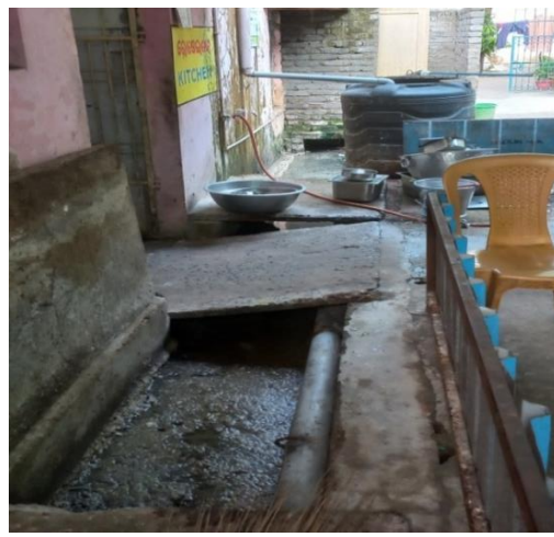
Blocked open drain, passing through the kitchen and washing area for utensils, at DHH, Bhadrak (30 May 2022)
