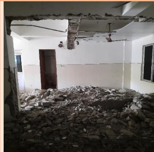
Dismantling of the OPD portion of the building, for extension of OPD (10 May 2022)
