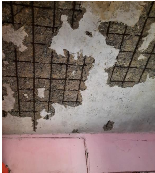
Ceiling of a residential quarter at PHC, Khuntagaon, not repaired (24 June 2022)
