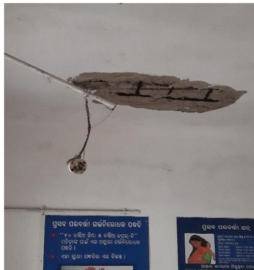
Dilapidated condition of the patient observation room at PHC, Khuntagaon (24 June 2022)
