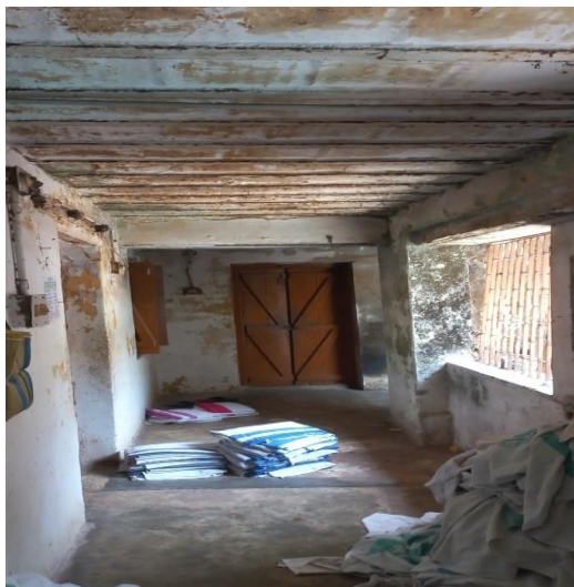
Dilapidated building used for storage of linens at DHH, Bhadrak (3 June 2022)
