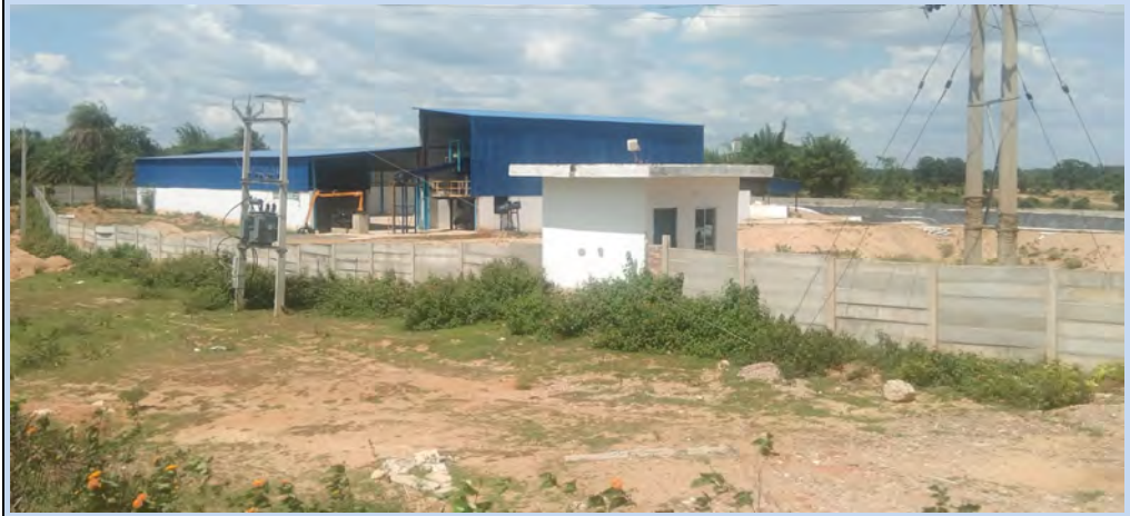
Exhibit 7.2 : Construction (including landfill site), at the Jhumritelaiya & Koderma cluster MC, without obtaining EC (photograph taken on 23 November 2022)
