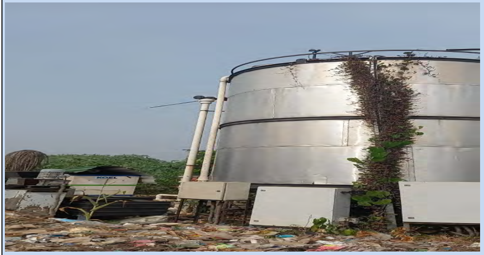
Exhibit 9.9: Idle bio-methanation plant at the Deoghar Municipal Corporation (photograph taken on 12 November 2022)
