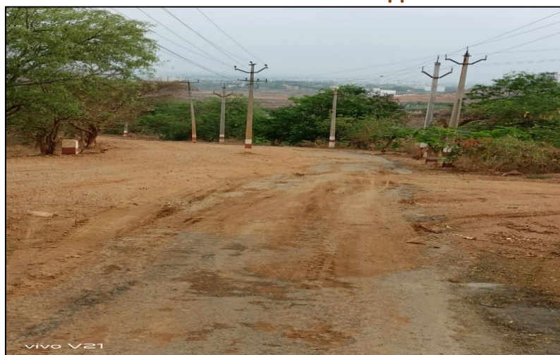
Picture No. 4.6: Poor condition of approach road
