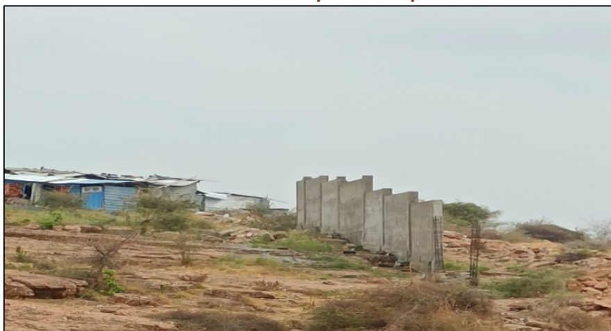
Picture No. 4.5: Incomplete Compound wall
