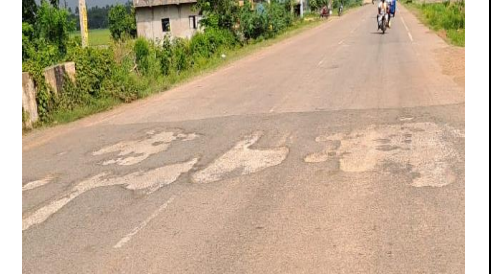
Photo No. 21: Pothole in SDBC on the roof slab of the box culvert
