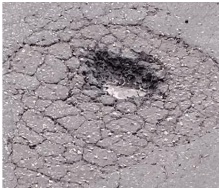
Photo No.12 : Pothole at RD 38.240 km of
