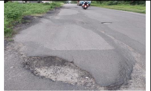
Photo No. 18: Depression at Km 26/125
