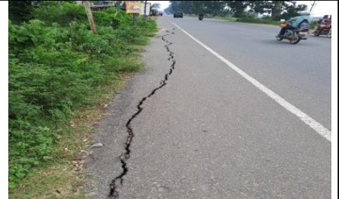
Photo No. 20: Liner and crocodile crack from Km 30/000 to Km 35/000
