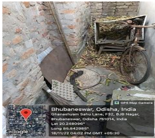
Photograph 25: Unauthorised encroachment over sewerlines, at BJB Nagar, Bhubaneswar
