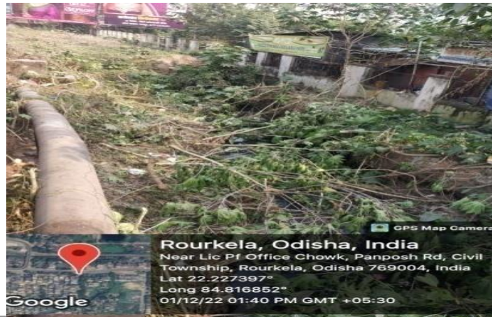
Photograph 20 : Non-maintenance of Drain at Raghunath Palli, Rourkela
