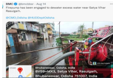
Photograph 14: Pumping of rain water at Satya vihar on 14 August 2022
