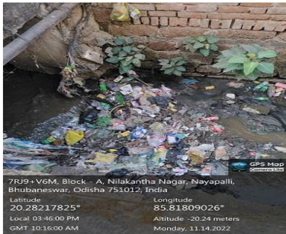
Photograph 24: Part sewerage of Ward No. 38, discharged in BMC Drain No. 10, near Nayapalli Nuasahi
