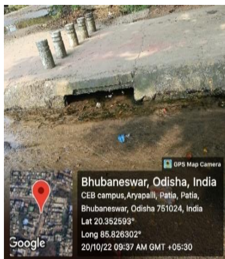
Photograph 10: Near Koil campus road, Patia-Nandankan road BMC
