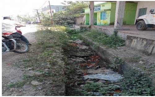
Photograph 18: Non-maintenance of Drain at Khetrajpur, Sambalpur
