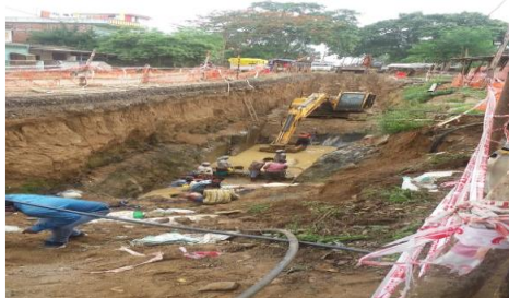
Photograph 26: Haphazard work at the Sambalpur sewerage project
