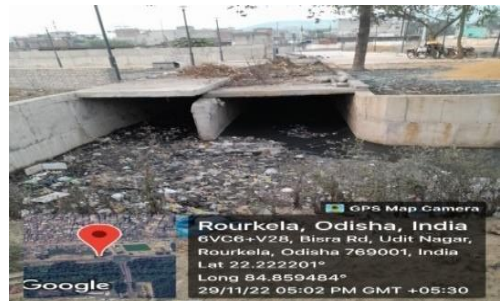
Photograph 43: Dumping of garbage in open drains, at the Bisra Road, Udit Nagar Rourkela
