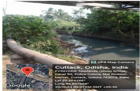
Photograph 19: Non-maintenance of Drain at Matrubhawan, Cuttack
