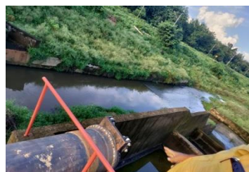
Photograph 58: Main drain I at Matagajpur flow to river Kathajodi
