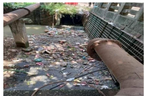
Photograph 6: Water supply pipe passing through the drain near Sreeleathers Patia, Bhubaneswar
