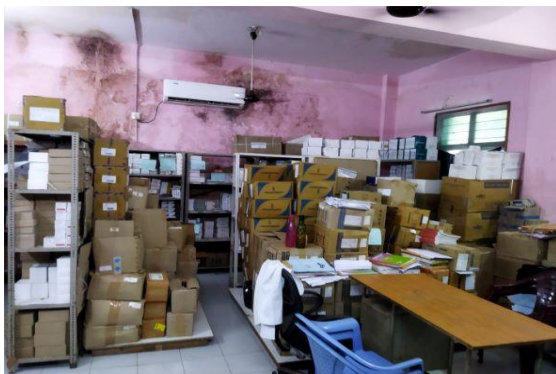
Figure 4.3: Seepage on walls in AH, Seethampeta (June 2022)
