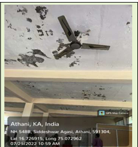
Picture No 5.12: Plastering falling off from roof at museum at Athani.
