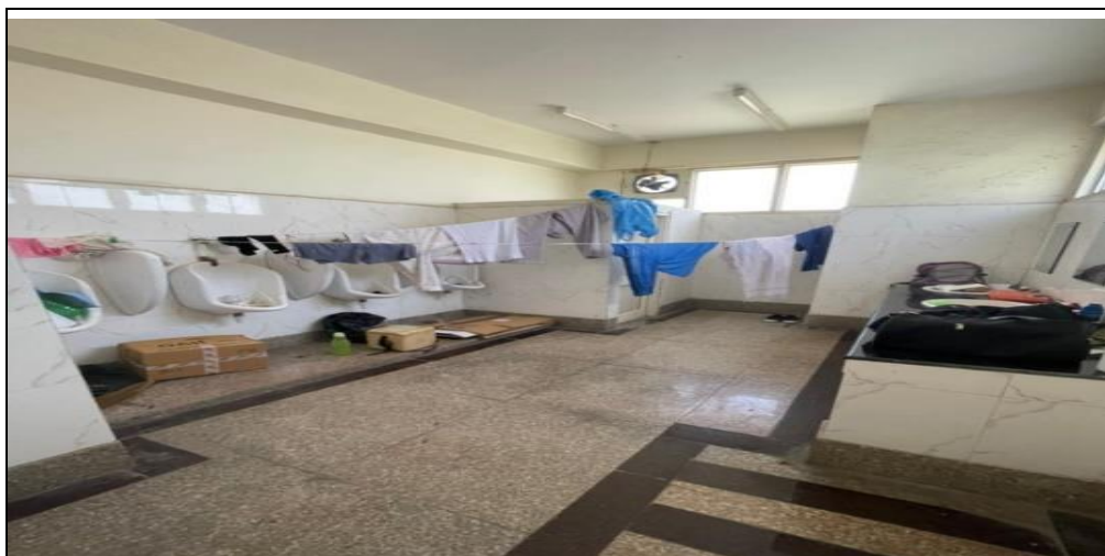
Laundry activities carried out in toilet at SDCH Samalkha (06 March 2022)
