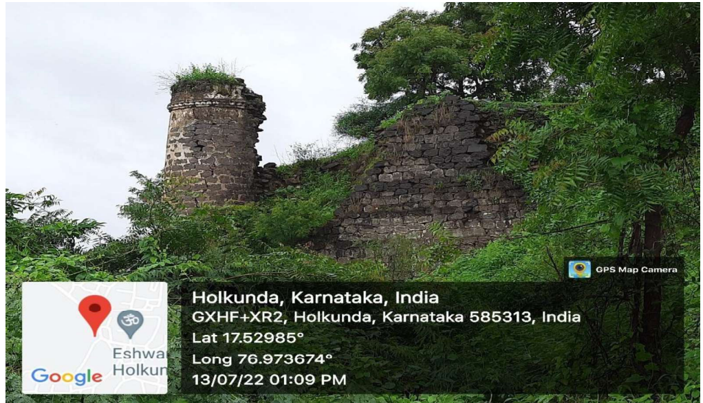
Picture No 2.1: The condition of Bahamani Tombs at Holakunda which require immediate conservation, Kalaburagi Taluk, Kalaburagi District.
