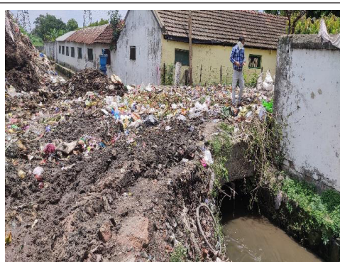
Fig 4.21: Dumping of solid waste on the approach road of the dumping ground of the Titagarh Municipality
