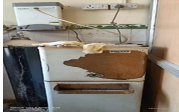
Non-functional water coolers in GFH, Haldwani, Nainital
