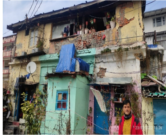
Dilapidated condition of residential quarters of DH, Nainital
