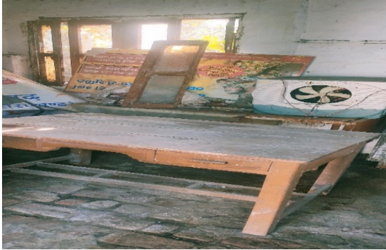
Sub Centre-Kaulagarh, Dehradun used as storeroom
