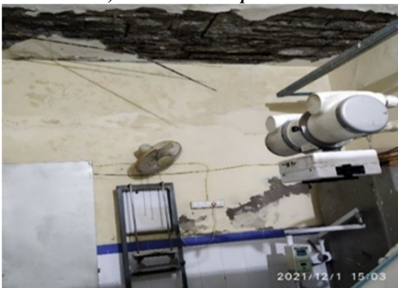
X-ray room in dilapidated condition at CHC, Doiwala, Dehradun
