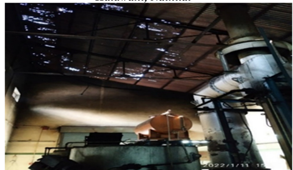
Dilapidated Tin Roof of CBWTF Haldwani, Nainital
