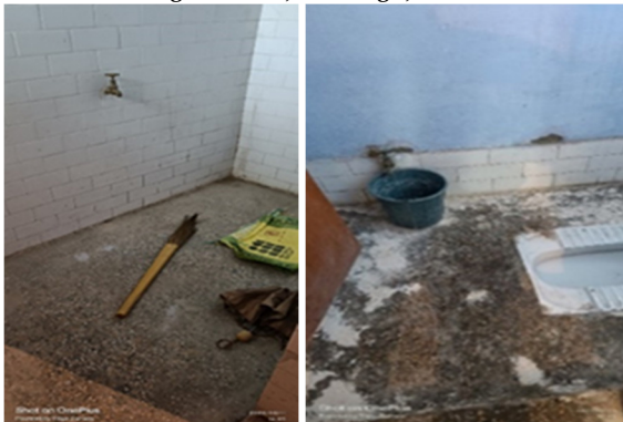
Unusable washroom and toilet due to lack of water in PHC, Chakalua, Nainital
