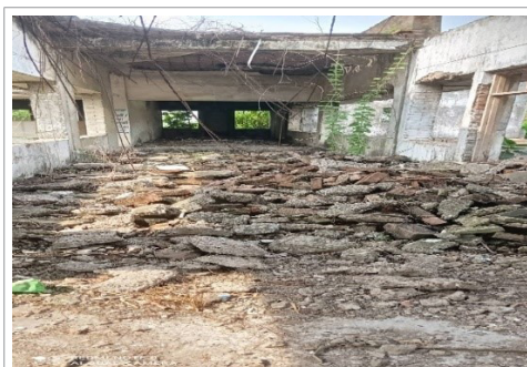
Images 6: Roof corridor of manufacturing plant of BVSL, at Industrial area, Hajipur (Vaishali)
