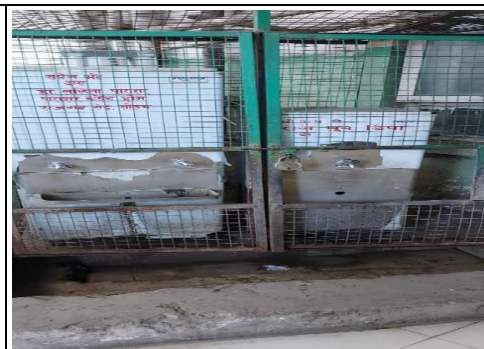
Picture 3.6: Non-functional water cooler in DH Solan
