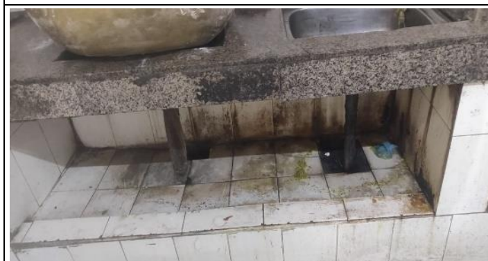
Picture 3.23: Sink in kitchen was found in broken and choked state in IGMC Shimla
