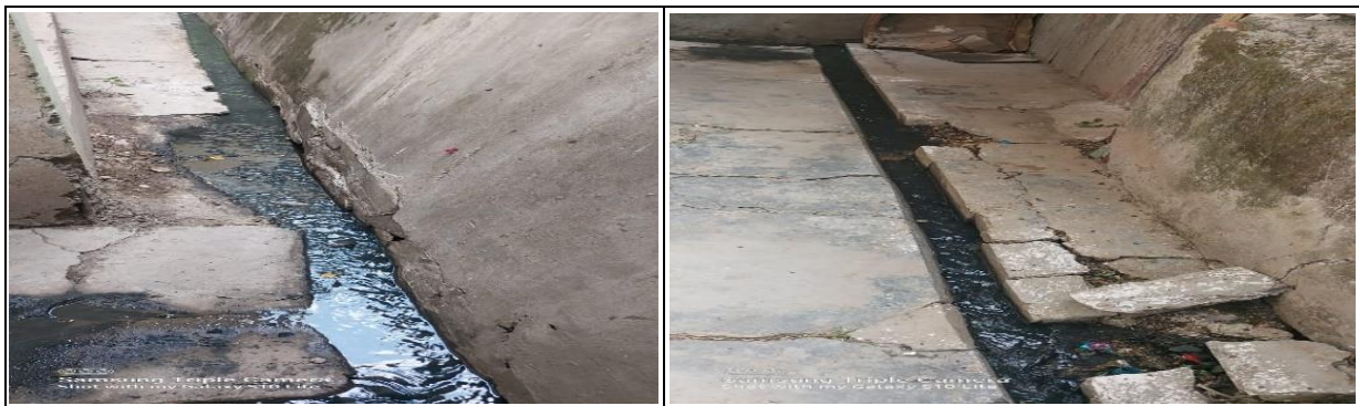
Pictures 3.41 and 3.42: Untreated wastewater let in public drain in IGMC
