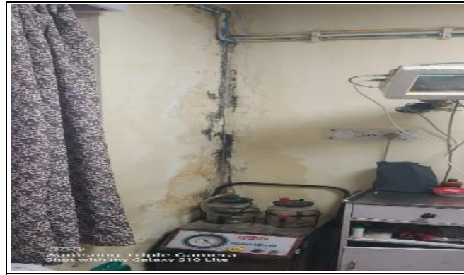
Picture 3.15: Seepage and dampness of the wall of CCU at IGMC Shimla.
