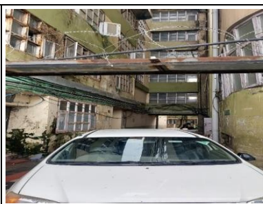
Picture 3.49: Old oxygen pipeline
