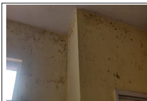
Picture 3.16: Dampness on the wall of main OT medicine store IGMC, Shimla
