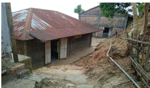
The approach road of Tuipang AWC, Tuipang ICDS Project was slippery during rainy seasons which was dangerous for children and pregnant women.
