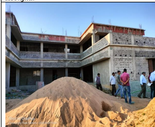
Image 5.2 : Incomplete Primary School Building at the Angulia R&R Colony, relating to the Kanpur Irrigation Project, Keonjhar
