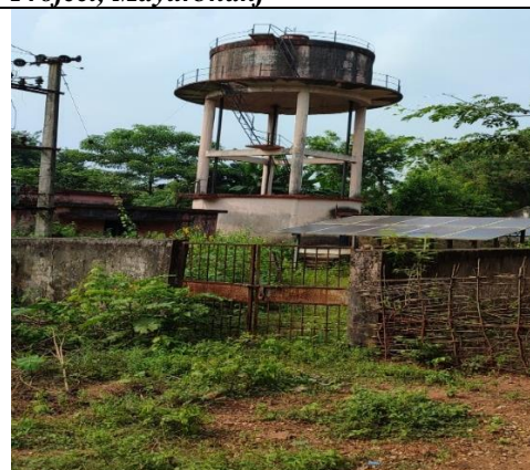
Image 5.3: Defunct Piped Water Supply System at the Rangamatia R&R Colony, relating to Subarnarekha Irrigation Project, Mayurbhanj
