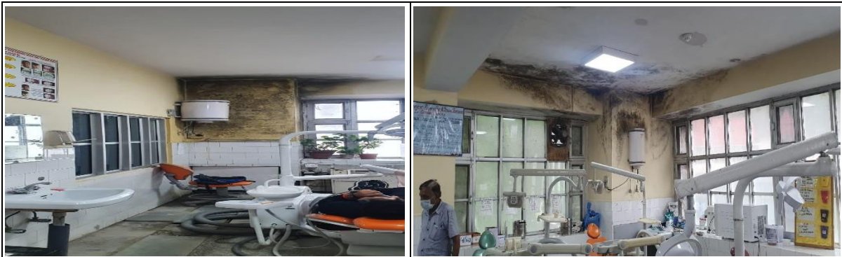
Pictures 9.1 and 9.2: Showing seepage in the walls.
