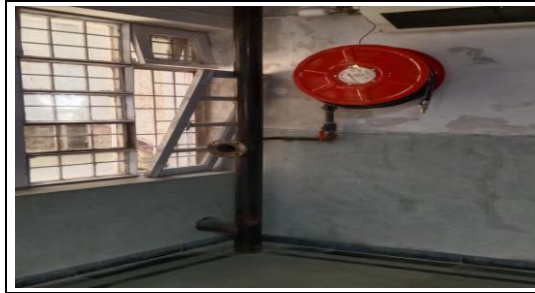
Picture 9.21: Incomplete Fire Hydrant at HHMH&R Shimla
