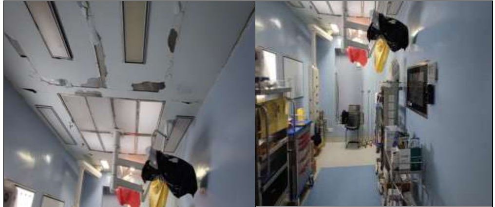
7. OT not in use in DKS PGI, Raipur due to seepage (Date 03 June 2022)
