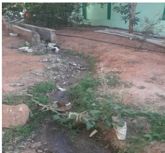
Photograph 3.1.11: Accumulation of waste water, due to partly constructed drainage system at the STGH, Tikabali HS, Tikabali Block, Kandhamal District
