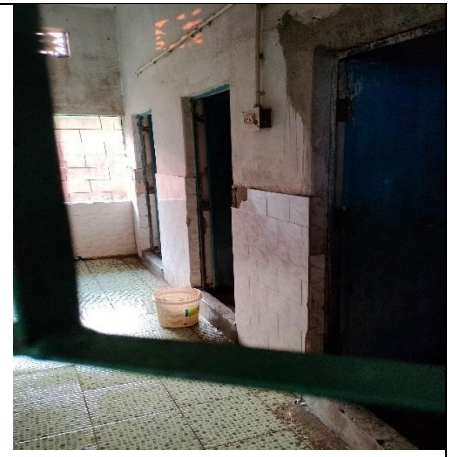
Photograph 3.1.7: Latrine door damaged at the STGH, Badgobra Ashram School under the Tiringi Block, Mayurbhanj District
