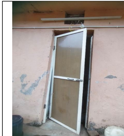
Photograph 3.1.6: Broken door of toilet of the STGH at Dogharia, Nuagada Block, Gajapati District
