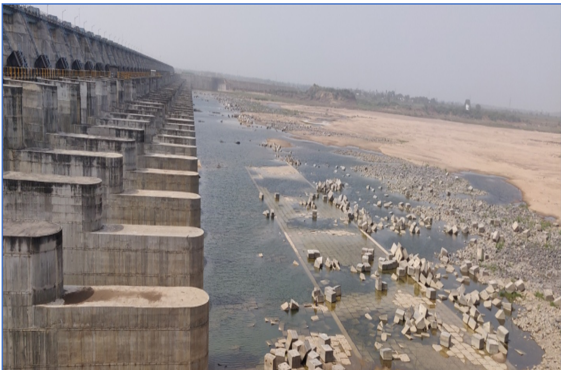
Figure 5.1 – Damaged CC Blocks and apron at downstream side of Annaram barrage
