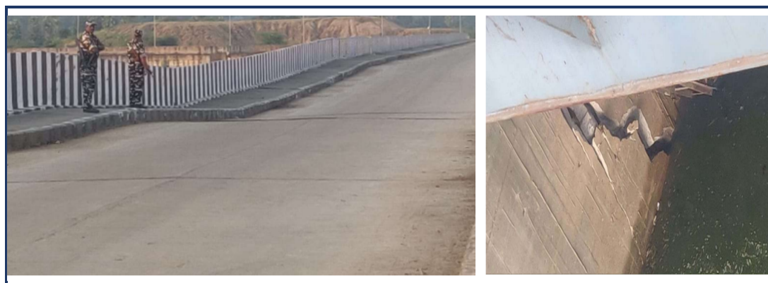
Figure 5.3 – Sinking of Piers of Medigadda barrage in October 2023
