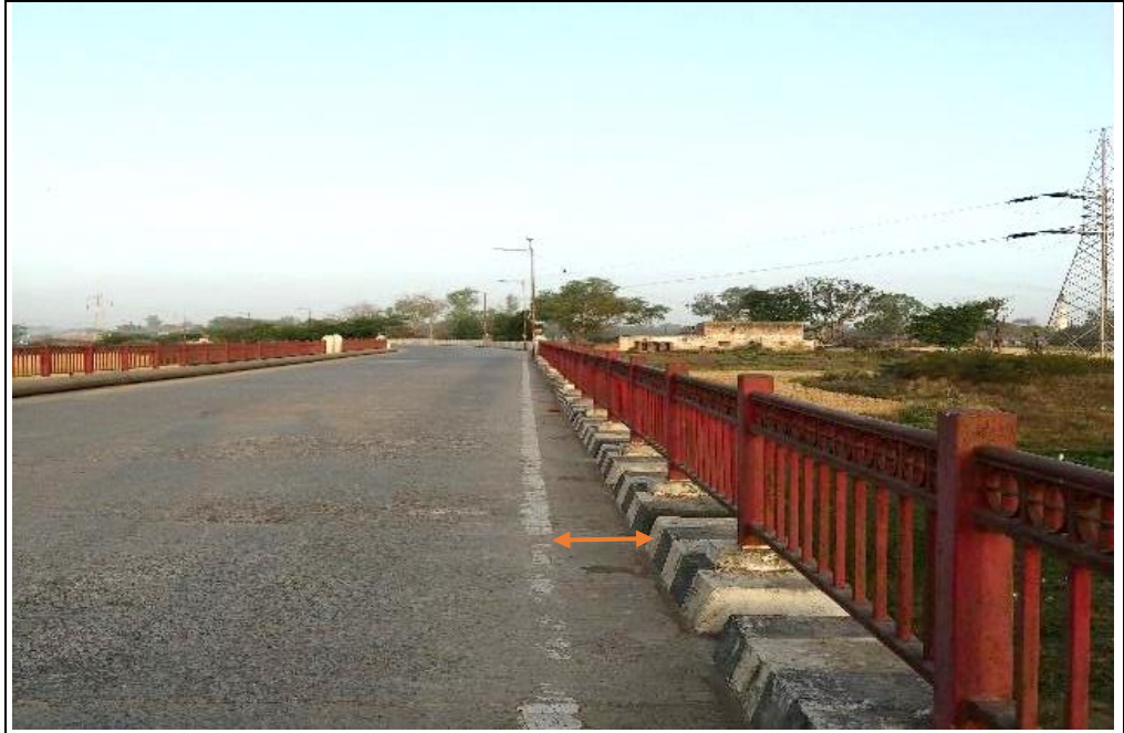
Submersible Bridge on Rinmukteshwar to Ranjeet Hanuman Road (Ujjain) with insufficient kerb width.
