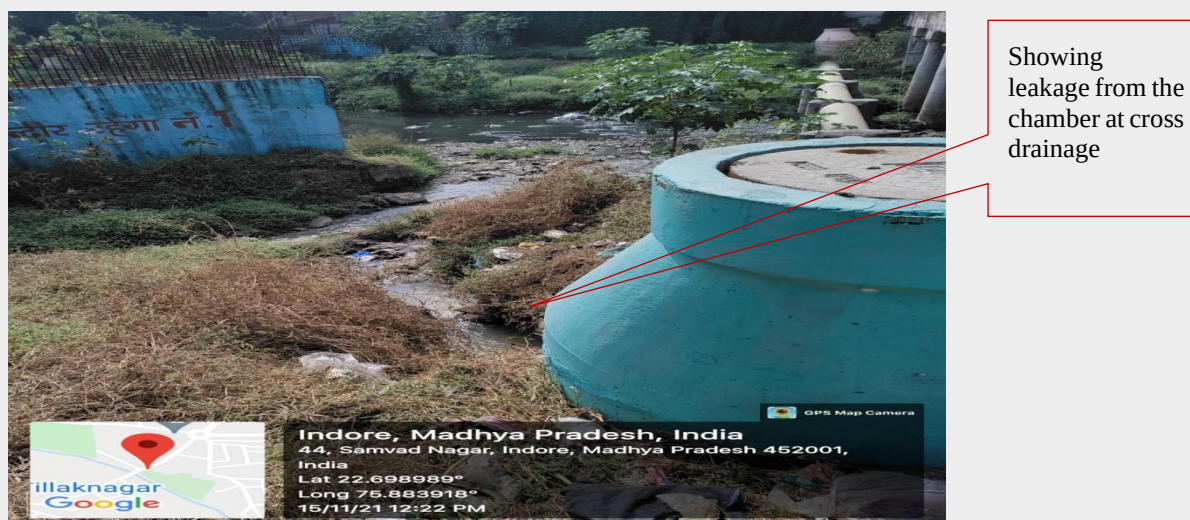
Images No. 2.10 and 2.11: Showing leakage from the sewerage pipeline in the nala Crossing
