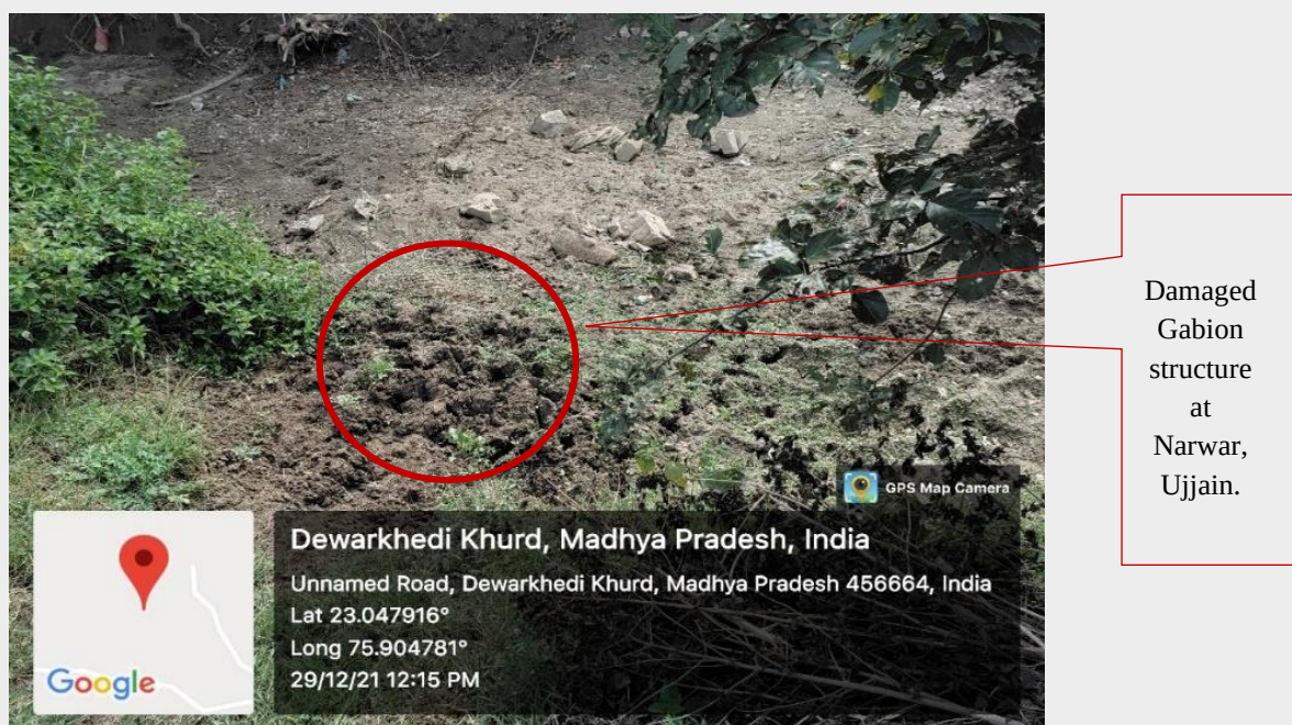
Image 6.4: View of damaged Gabion structure at Harnvada village
