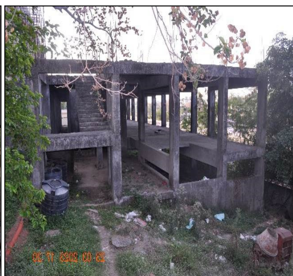
Picture No. 2.2: Incomplete structure adjacent to Block-E
