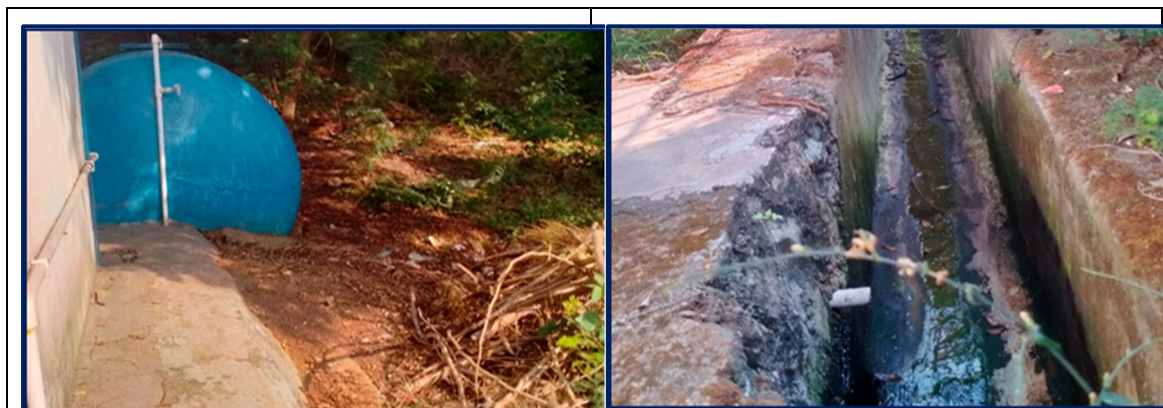
Picture 7.5 – Treated Water from Sewage Treatment Plant discharged into Main Drain
