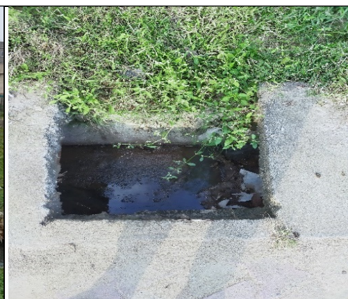
Picture 4.11: Stormwater drain filled with sewage
