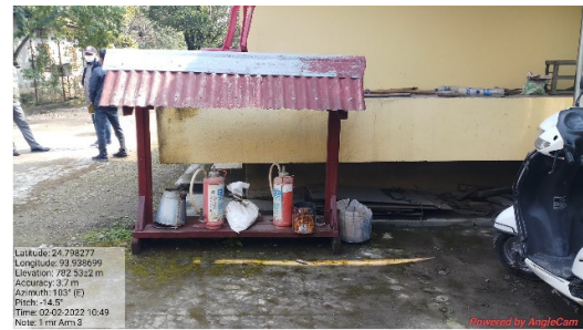
Sand buckets without sand and expired fire extinguishers (1 st Battalion Manipur Rifle)
