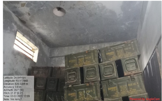
Water leakages in the Arms KOTE ( 7 th Battalion Manipur Rifles)
