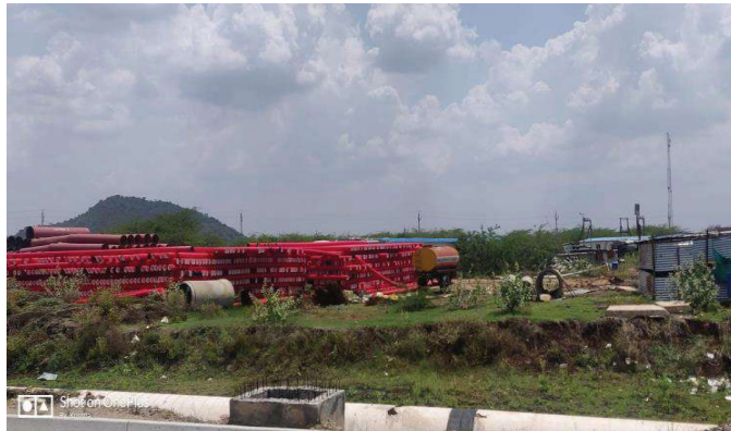
Picture 3: Pipes lying idle at Water Treatment Plant (Package XV)
