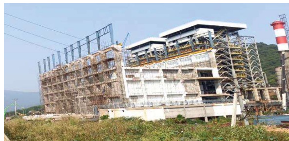
Picture 5: Jindal waste to energy power plant, Kapuluppada
