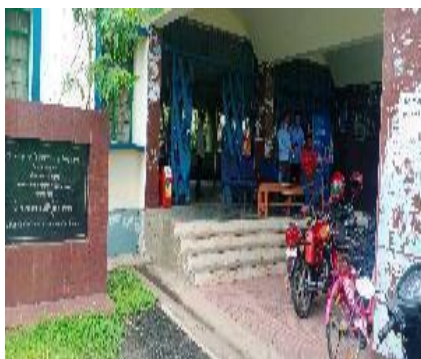
Picture 2.1: No ramp at the entrance to Dr. Meghnad Saha Institute of Technology, Haldia, Purba Medinipur
