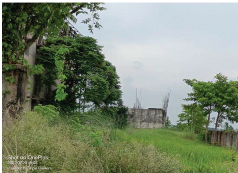
Fig. 2.9: Dilapidated condition of the incomplete CFC of the Re-rolling Mills Cluster, Jagatballavpur, Howrah
