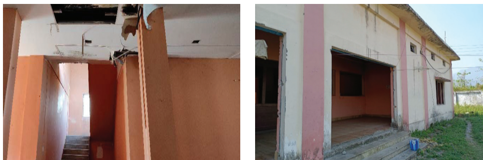
Fig. 2.20 and Fig. 2.21: Building in dilapidated condition with damaged roof, stolen doors etc.
