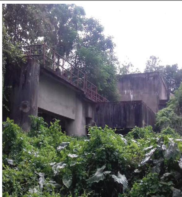
Fig. 2.12: Dilapidated condition of Water Treatment Plant
