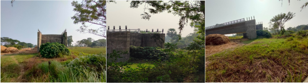
Photo No. 14: Source: Photos taken during Joint Inspection (February 2023) showing the completion of HL Bridge and non-construction of approach road.
