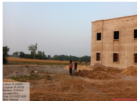
Photo No. 8: Construction of 180 capacity male ward of Bhadrak jail without outer jail wall
