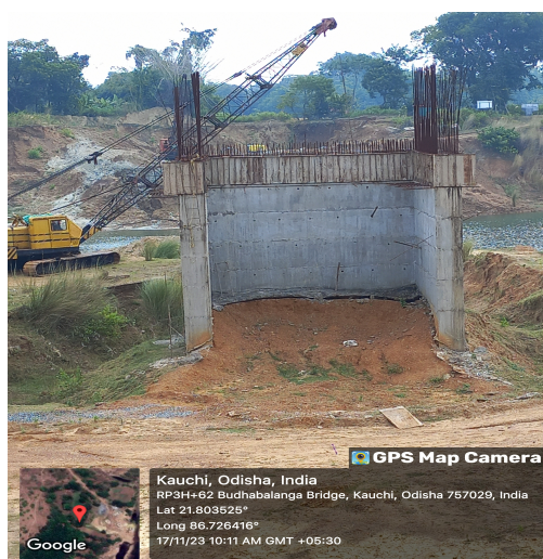
Photo No-7: Incomplete H.L Bridge over Budhabalanga river (Mayurbhanj R&B)
