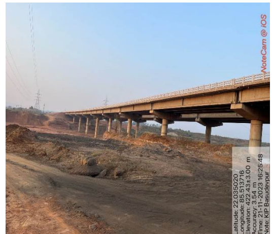
Photo No. 13. Incomplete bridge work over Spill Channel at Chainage 173.325 km of Rimuli-Roxy-Rajamunda section of NH-215 (New NH 520)
